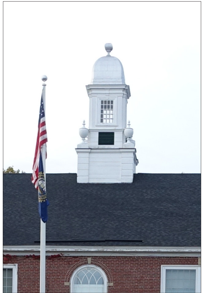
Roof features, such as bell towers, can often be found on institutional buildings.
