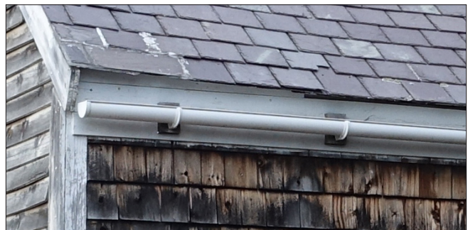
The half-round gutter collects stormwater as it runs down the roof surface.
