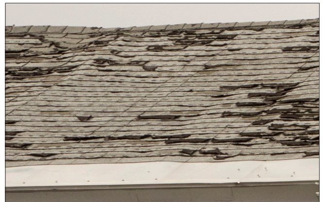
This 3-tab asphalt shingle roof has exceeded its useful life. Given the unevenness of the surface, it would be prudent to have the underlying framing and sheathing reviewed by an architect or engineer prior to re-roofing.
