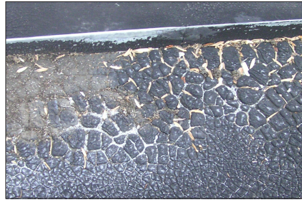
Rubber roofing systems can crack, eventually forming leaks. Significant cracking of this roof suggests replacement might be prudent.
