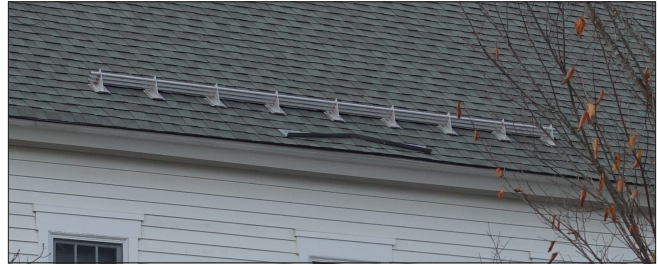
Snow guards prevent snow from sliding off a roof and are usually installed along a roof edge and are more prevalent above entrance doors.
