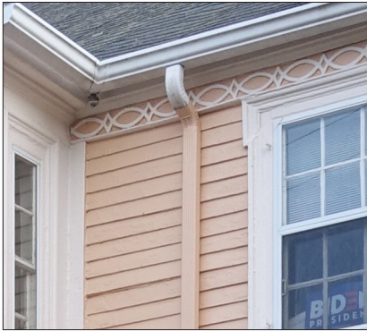
This downspout was painted to match the wall color, minimizing its visibility.
