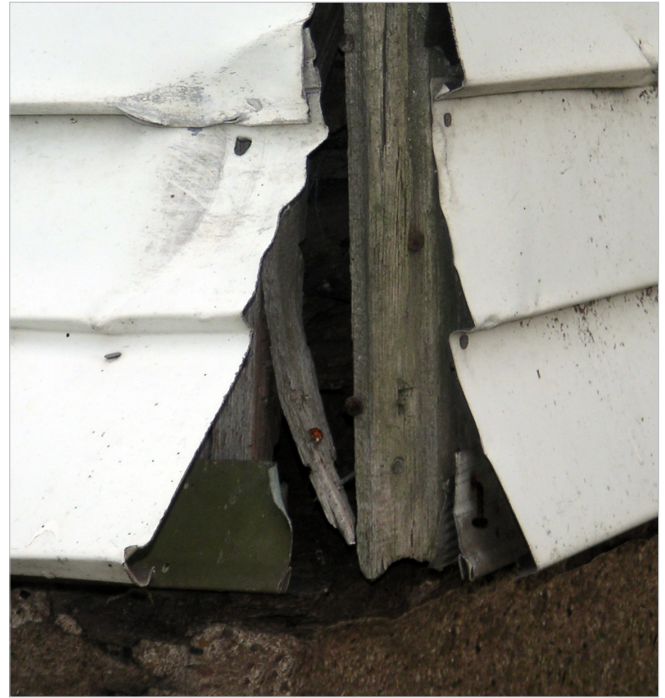
Aluminum and vinyl siding were sometimes installed to conceal an underlying problem. In some cases, removal might be necessary to repair a deteriorated condition.
