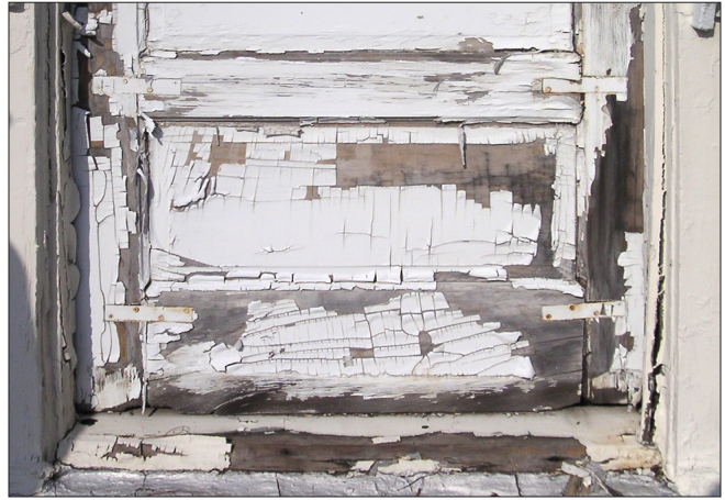
The paint on this door has alligatored, and severe cracking is visible. Removal of paint down to bare wood and proper door repair are recommended prior to repainting.
