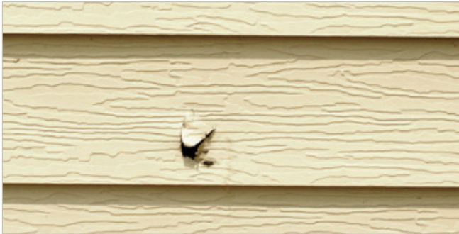
Replacement of this aluminum siding is the best way to repair this puncture. A wood-grained texture is inappropriate.
