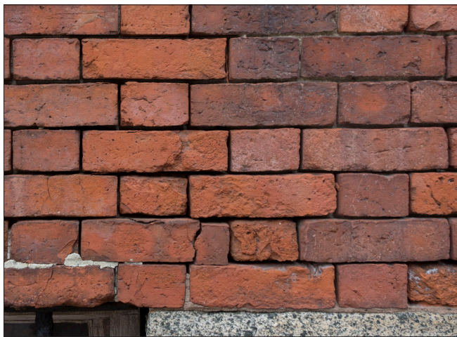
The mortar has weathered from most of the brick joints, reducing the structural capacity of the wall. The surface of some bricks has spalled, and a settlement crack has developed near the corner of the window.
