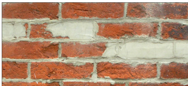
The rough texture and uneven surface suggest an aggressive cleaning method was used. Stucco patches replace bricks and efflorescence, a white powdery substance, can be seen on the surface.
