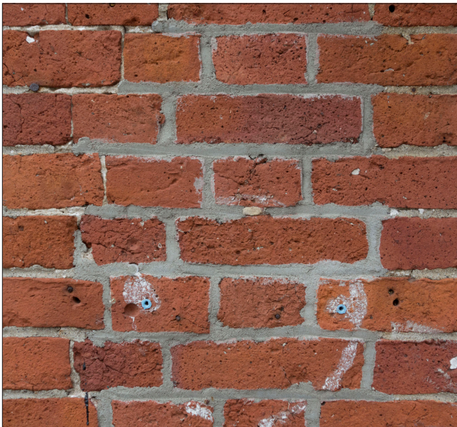
The central bricks have been repointed with what appears to be a Portland cement mortar that is harder than the hand-made brick. In addition, the mortar color and tooling poorly match the original mortar.
