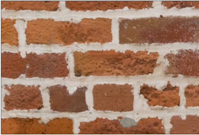
A saw was used to cut out the joints during repointing, thereby extending the vertical joints and damaging the bricks. In addition, both the vertical and horizontal joints have been widened.
