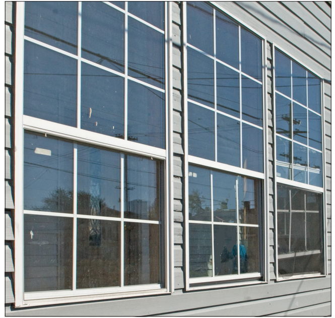
Vinyl windows with applied muntins lack the profiles and details of traditional wood windows and are not appropriate at historic buildings. They are also mounted flush to the outside wall without trim or casings.
