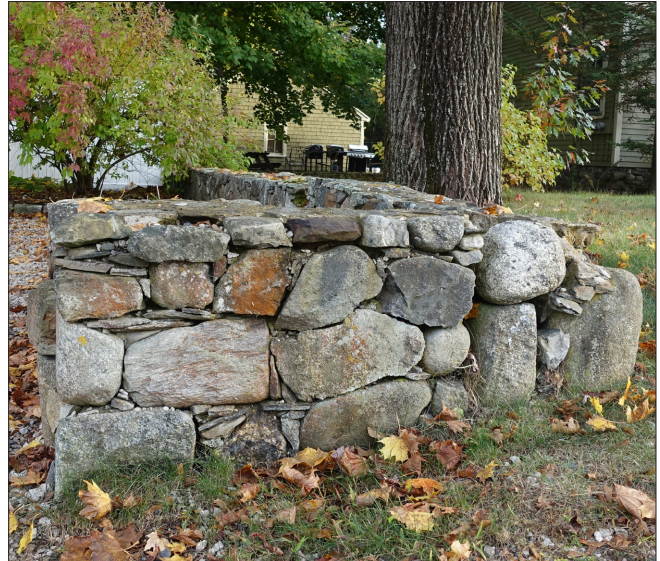
The dry-laid stone wall has smaller stones wedged between larger stones without the use of mortar.
