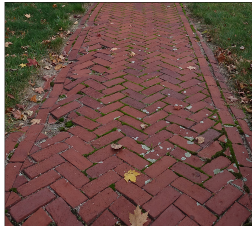
This brick walkway has a herringbone pattern with a running-bond boarder providing a formal entrance using a traditional material.
