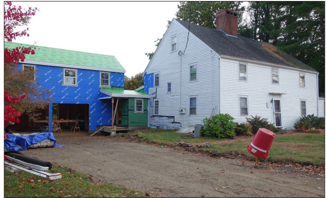
The new addition, located towards the rear, is both compatible with the historic house and contemporary in design. The smaller massing clearly identifies the addition as a secondary building. The volume, the roof slope and window openings match the historic residence.
