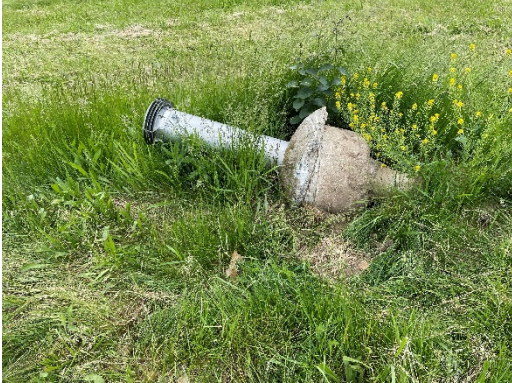
Photo #1 - Damaged gas vent in May 2021.
