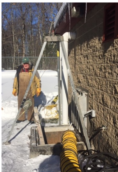
(Roger Philbrick at Church Road Pump Station 2/12/2021)
