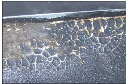
Rubber roofing systems can crack, eventually forming leaks. Significant cracking of this roof suggests replacement might be prudent.
