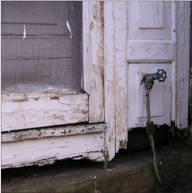
Leaking plumbing, including exterior hose bibs, can regularly expose woodwork to moisture, eventually resulting in rot. Wet wood can also be a desirable home for pests such as termites.
