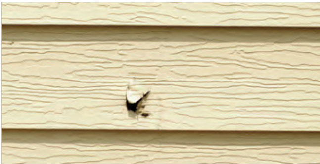
Replacement of this aluminum siding is the best way to repair this puncture. A wood-grained texture is inappropriate.
