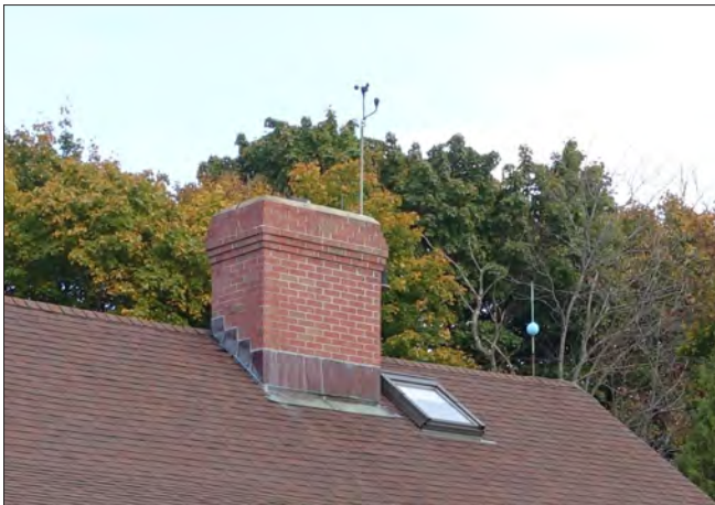
The skylight has a low profile and parallel to the roof slope, minimizing its visibility. Also note the stepped copper flashing at the brick chimney.
