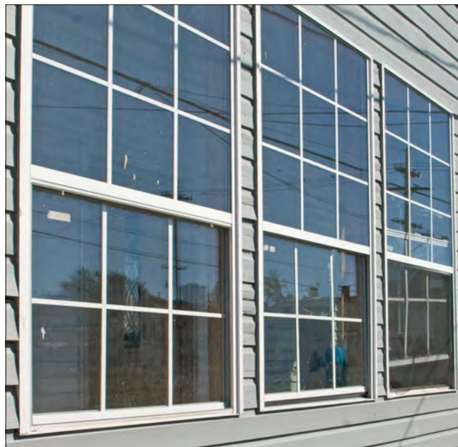
Vinyl windows with applied muntins lack the profiles and details of traditional wood windows and are not appropriate at historic buildings. They are also mounted flush to the outside wall without trim or casings.
