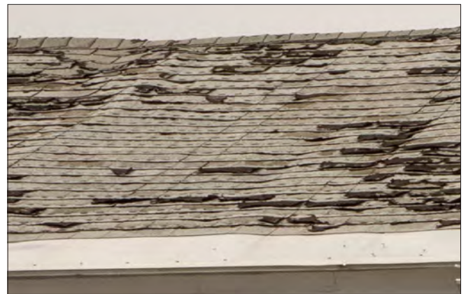
This 3-tab asphalt shingle roof has exceeded its useful life. Given the unevenness of the surface, it would be prudent to have the underlying framing and sheathing reviewed by an architect or engineer prior to re-roofing.
