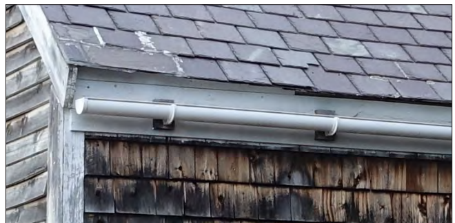
The half-round gutter collects stormwater as it runs down the roof surface.
