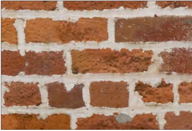
A saw was used to cut out the joints during repointing, thereby extending the vertical joints and damaging the bricks. In addition, both the vertical and horizontal joints have been widened.
