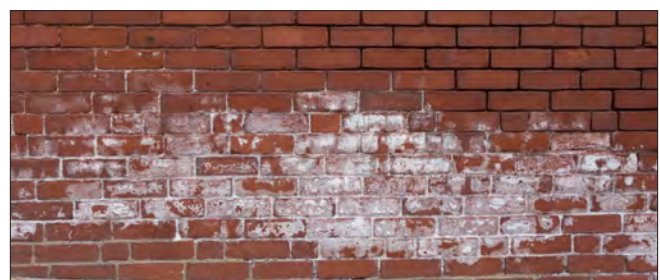
Efflorescence, or white bloom, is an indication of moisture in the wall. There is a lack of mortar at the upper right.
