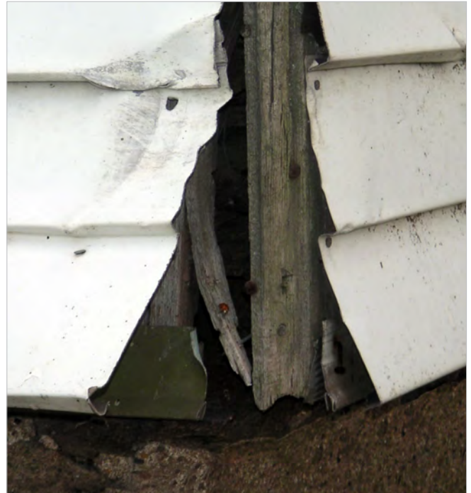
Aluminum and vinyl siding were sometimes installed to conceal an underlying problem. In some cases, removal might be necessary to repair a deteriorated condition.
