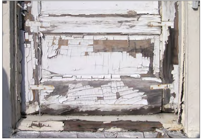
The paint on this door has alligatored, and severe cracking is visible. Removal of paint down to bare wood and proper door repair are recommended prior to repainting.
