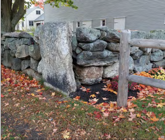
Granite, which is readily available in Rye, is a very durable material that is ideal for the construction of landscape walls. This dry-laid granite wall includes larger stones held in place by smaller ones, all topped by a relatively flat capstone.
