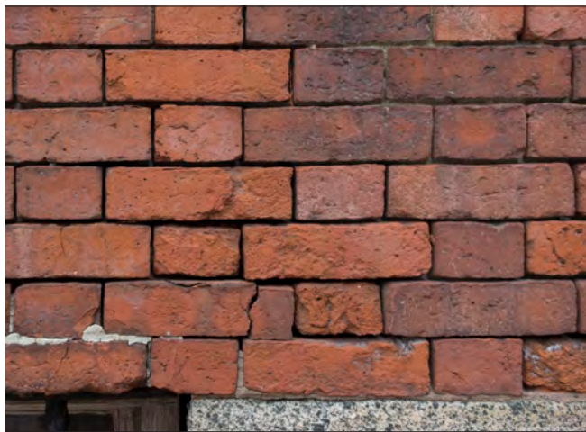
The mortar has weathered from most of the brick joints, reducing the structural capacity of the wall. The surface of some bricks has spalled, and a settlement crack has developed near the corner of the window.
