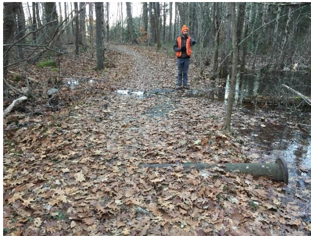
Drainage devices help keep trails dry. This culvert is partially exposed however.
